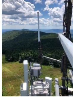
A Band Class 14 transceiver was installed on a tower at Mt. Snow in July.
